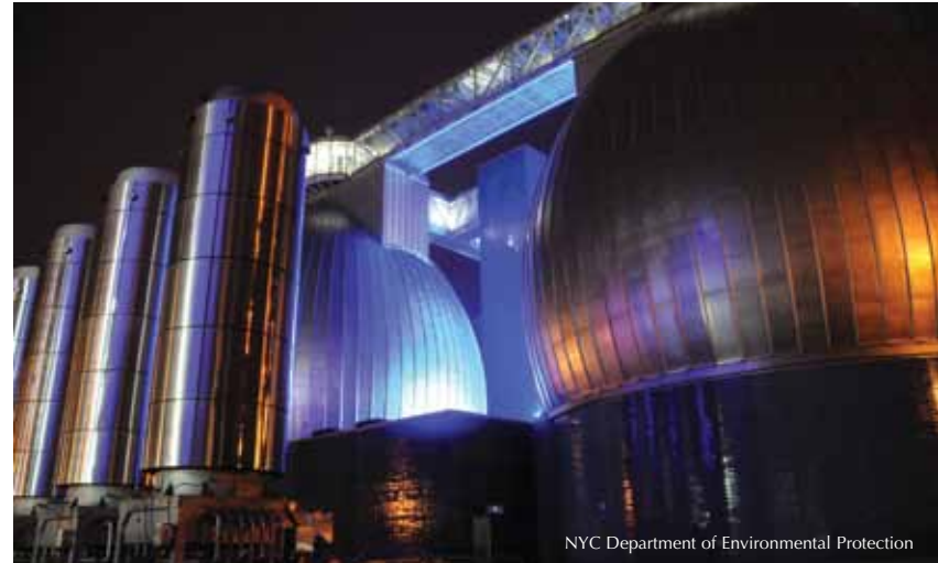
Newtown Creek Wastewater Treatment Plant in Greenpoint, Brooklyn. The lighting scheme, designed by L'Observatoire International, subtly casts a halo of blue light around the 145-foot-high, stainless steel-clad eggs, which process as much as 1.5 million gallons of sludge every day.
